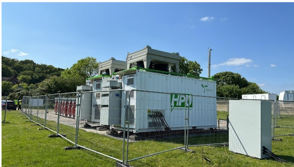
Hydrogen generators used on BBC SpringWatch. Source: GeoPura
