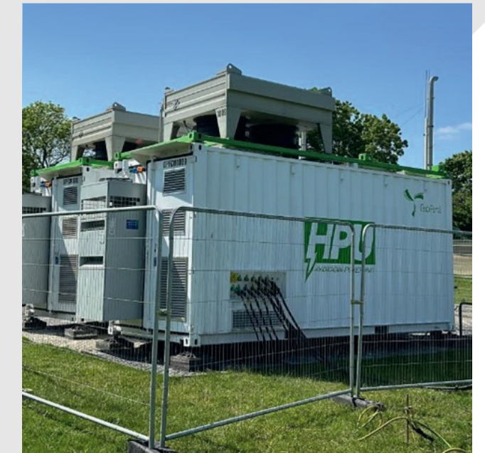
Hydrogen generators used on BBC SpringWatch. (Source: GeoPura )
